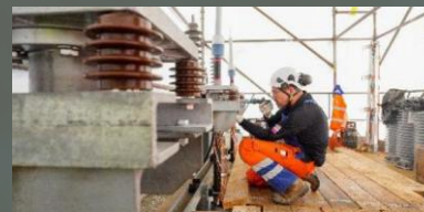
Lochem – expansion and transformation to an MV and HV facility
